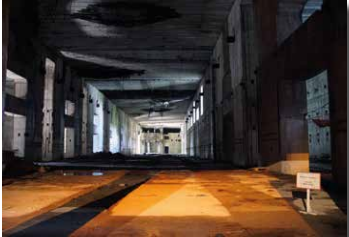
Bunker Valentin, impact de bombe (2015)
